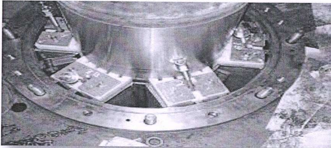
Francis Turbine At Regular Maintenances
